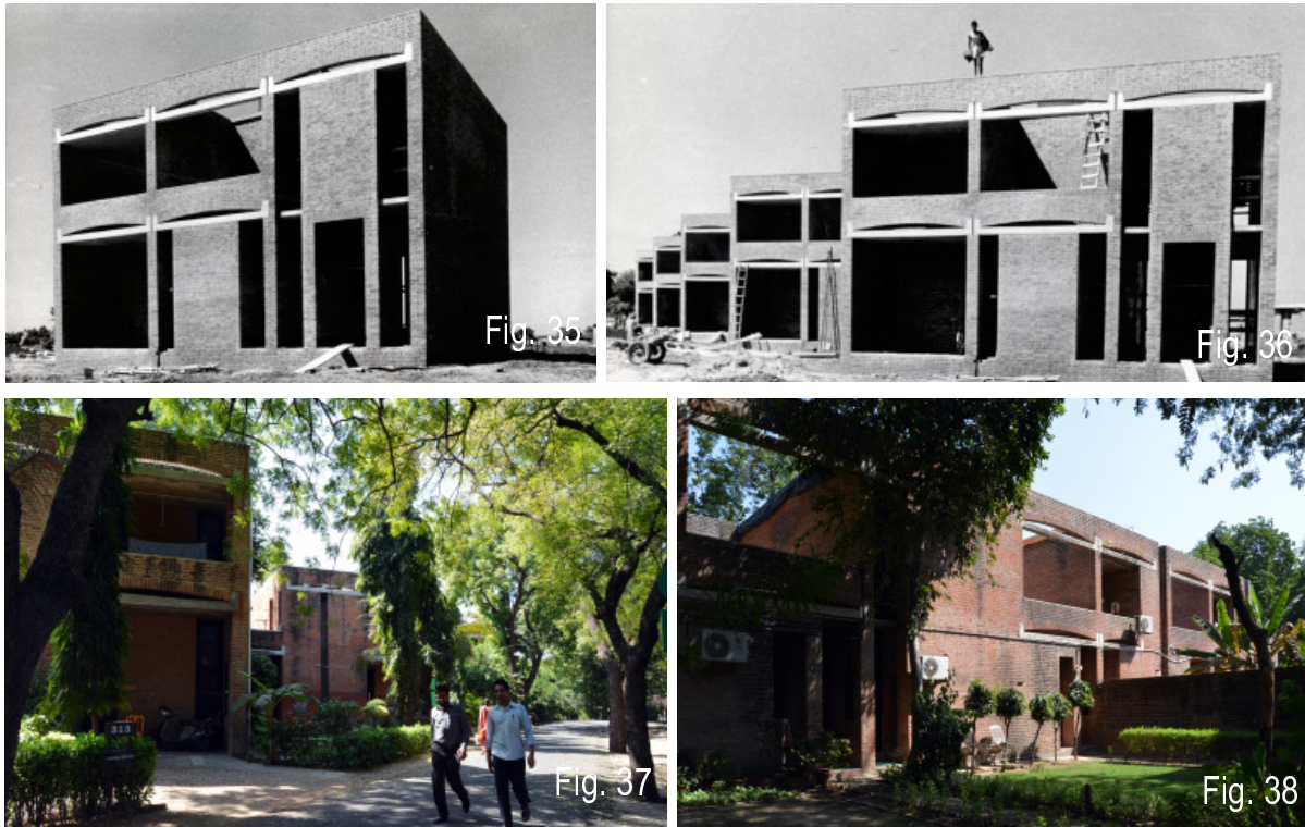
Houses for Faculty -- Fig. 35 (Top Left): The first Type 5 House : Fig. 36 (Top Right): A row of Type 4 houses Figs. 37, 38 (Bottom): Type 3 houses
