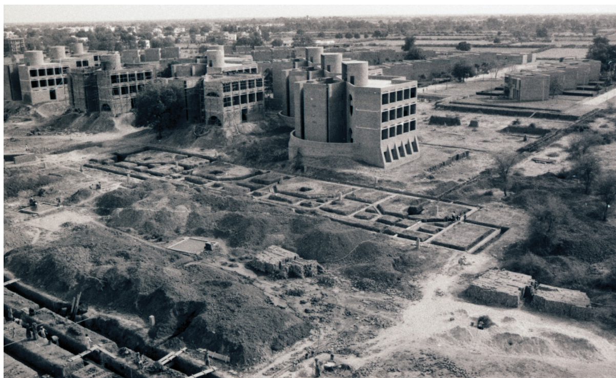
Fig. 1: A view of the site during construction. Foundation work for the Classrooms and Faculty Wing is in progress
