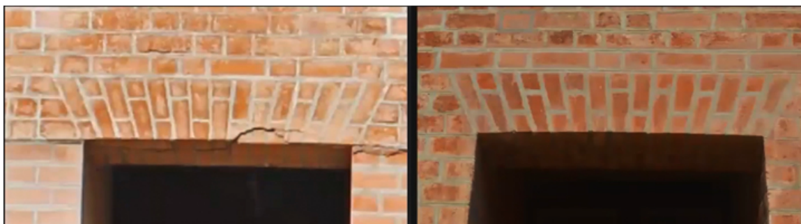
Vikram Sarabhai Library, showing brick restoration. Note: The same bricks are used in the dormitories
