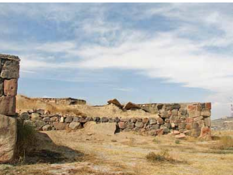
Ruinous state of the surrounding walls
