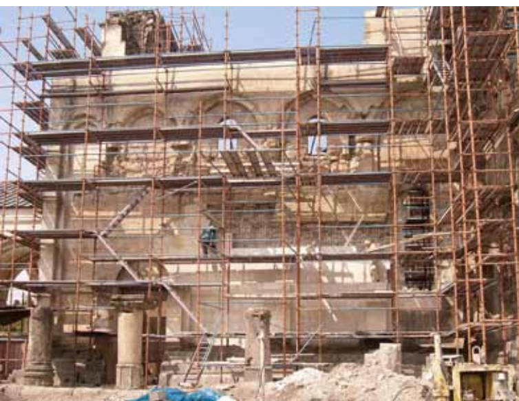
Restoration of the wall facing by means of a metal net and cement mortar
