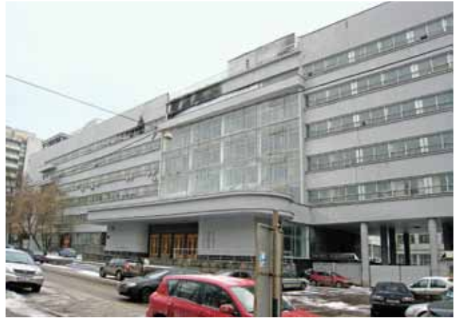
In 2006 a fire destroyed the top floor of the Pravda newspaper building (1931–37, P. A. Golosov). Two years later nothing had been done to prevent further decay. Situation in 2008 (photo: A. Zalivako)
