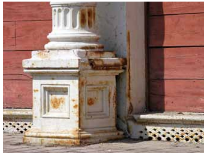
Galveston, cast iron damage
