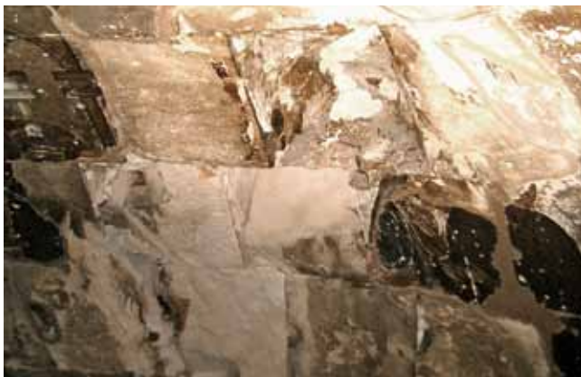
Sioni Church, vault of the south conch with fallen-off cap stone: the mortar shows an imprint of the lost stone trapezoidal in its cross section (photo: Barthel & Maus)
