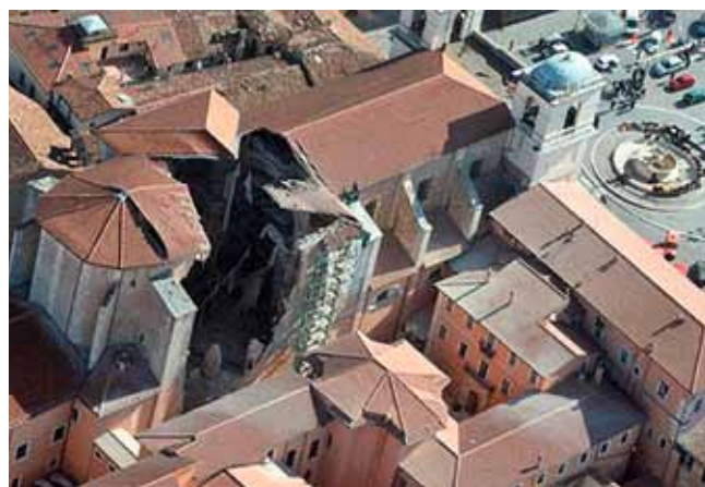
L'Aquila, aerial view of the damaged cathedral
