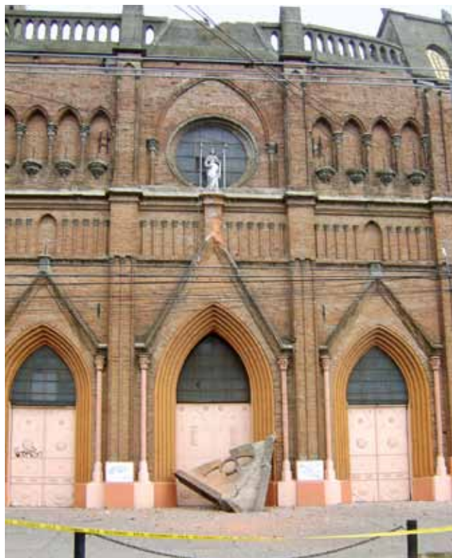
Corazon de Maria, damaged church
