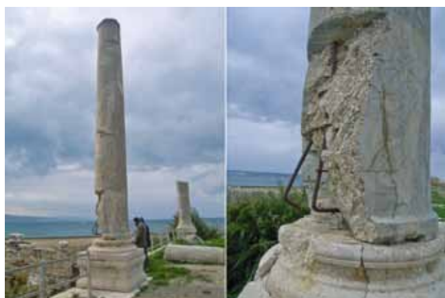
Exposed steel reinforcements from previous reconstructions. Columns could be struck by lightning during storms and thus be destroyed further
