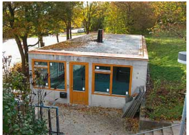
Gatekeeper's house with copper edging to the roof and highly reflective blue windows on the façades 2010 (photo: Monika Maus)
