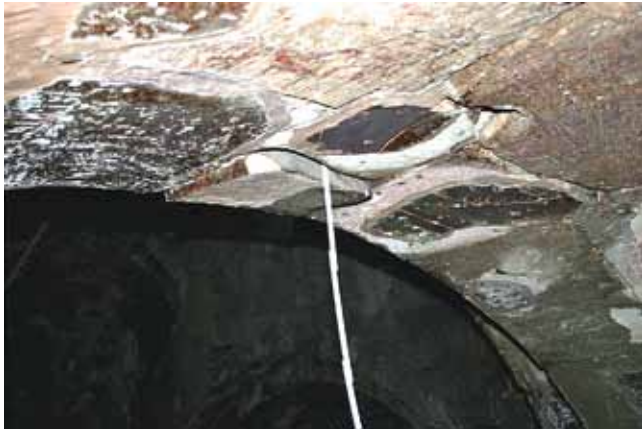
Sioni Church, cap stone in the vault of the south conch: the stone has sunk 30 mm (photo: Barthel & Maus)
