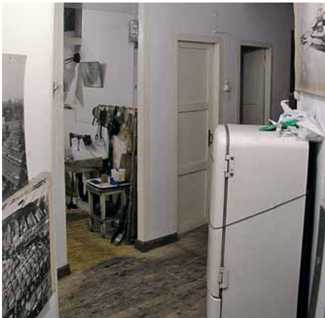
Melnikov House and Studio, floor damages, 2009 (photo: A. Deill).
