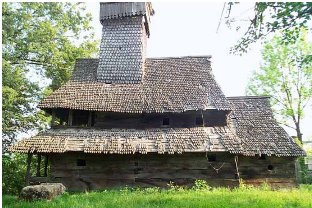
Roof damage on the south side of the church in Kolodne (photo: A. Kutnyi)
