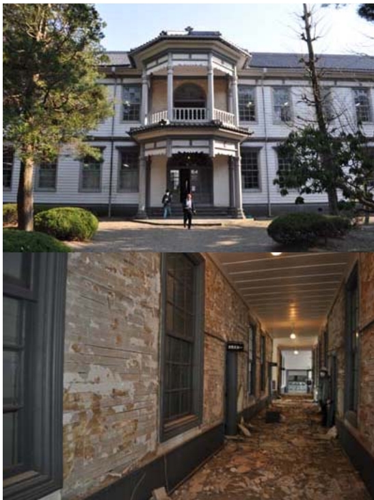
Figure 2.9 Damage to the important cultural property, Fukushima Prefecture Jinjo Junior High School (Top: Building exterior; Bottom: Peeling lath wall)
