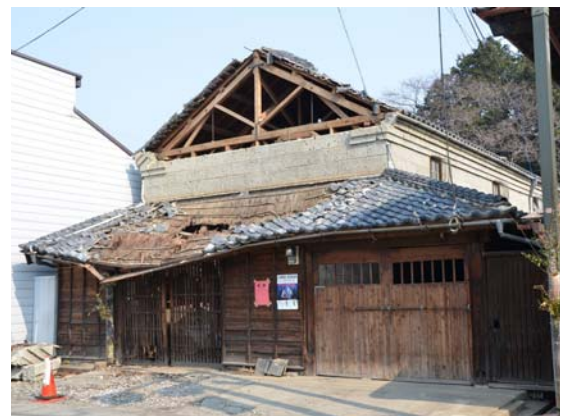
Figure 2.26 A damaged house in Makabe
