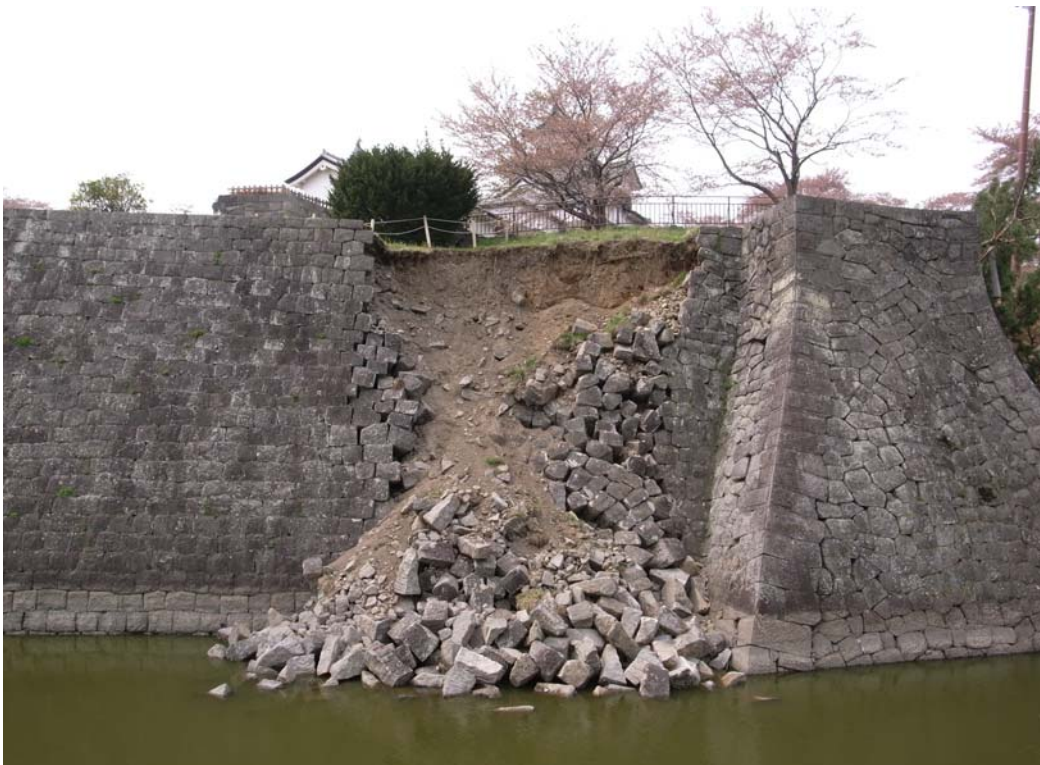
Figure 2.30 Collapsed masonry walls of Komine Castle
