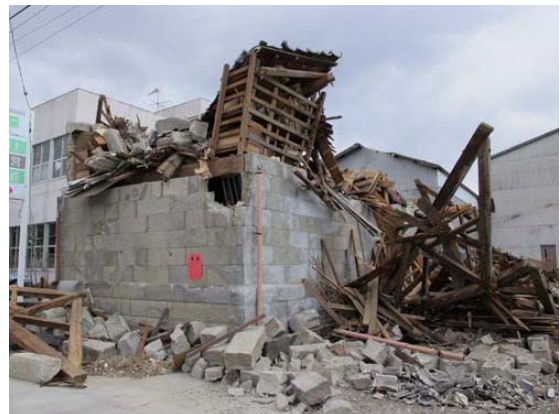
Figure 2.14 Collapse of stone storehouse in Makabe, an Important Preservation District for Groups of Traditional Buildings
