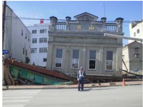
Figure 2.13 Tsunami-caused damage to the registered tangible cultural property, the Otokoyama Shuzo original store
