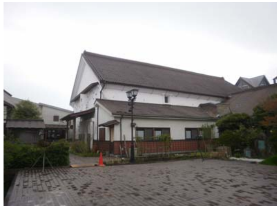
Figure 4.3 Collapsed stone gable wall
