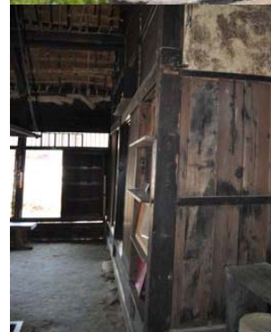
Figure 2.8 The important cultural property, the former Baba Family Residence, which is tilting (Top: Exterior; Bottom: Tilting interior)
