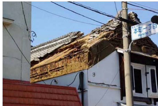
Figure 2.10 Damage to classic dozo (mud-wall warehouse) - the registered tangible cultural property, the Mori Goshi Gaisha storehouse
