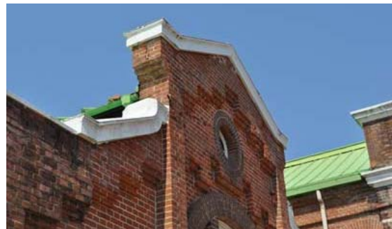
Figure 2.22 Disaster-affected Chateau Kamiya winery building, an important cultural property (Top: Building exterior; Bottom: Cracked gable wall)
