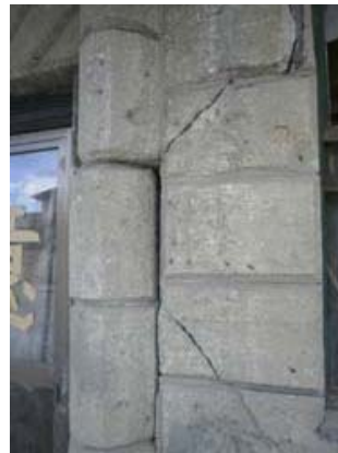
Figure 2.15 Damage to the Takahashi Family Residence, a registered tangible cultural property
