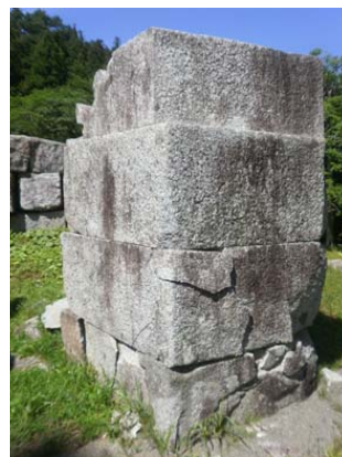
Figure 2.16 Displaced and cracked stone masonry at the Hashino Blast Furnace, a historic site in a Kamaishi City
