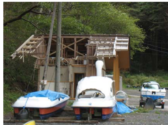
Figure 2.35 Facilities destroyed by the tsunami (Jodogahama)
