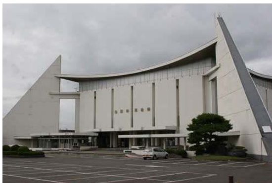
Figure 2.23 Furukawa Civic Hall which underwent damage to its non-structural components (from Furukawa city homepage 3) )
