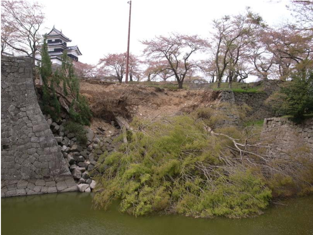
Figure 2.29 Collapsed masonry walls of Komine Castle
