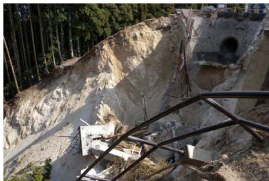
Figure 2.24 Ishioka Electric Power Plant (Top: Before earthquake; Bottom: After earthquake) (Ishioka city, Ibaraki Prefecture)
