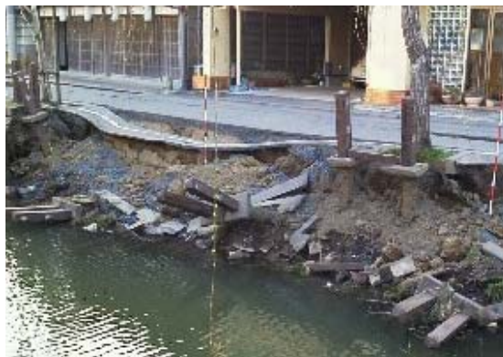
Figure 2.28 Historic riverside damaged
